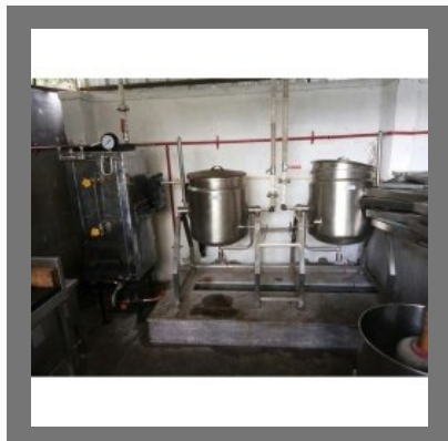
Steam Boiler Plant
