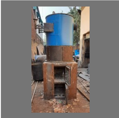
Thermic Fluid Heater
