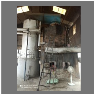
Used Thermic Fluid Heater
