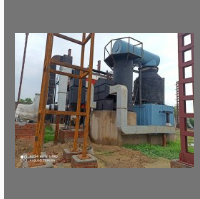
Woodcoal Fired Thermic Fluid Heater
